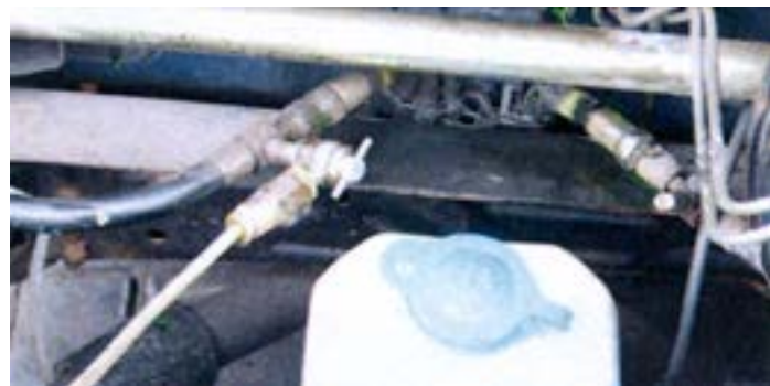
Figure 2: Two valve connection points.
